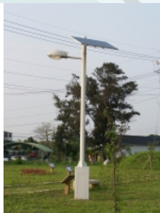
Solar-powered LED Streetlights
